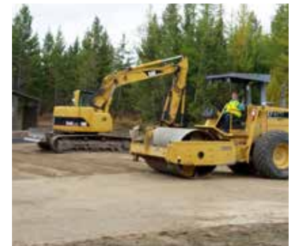
Several students from FVCC got real world experience building the new trailhead at Emmons Saddle as part of the Heavy Machinery certification program.
